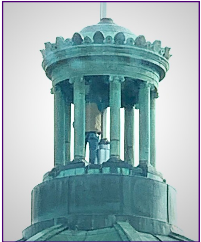
Garry Pluemer, Facilities and Maintenance Manager, attempting to thread a new rope in the dome.
